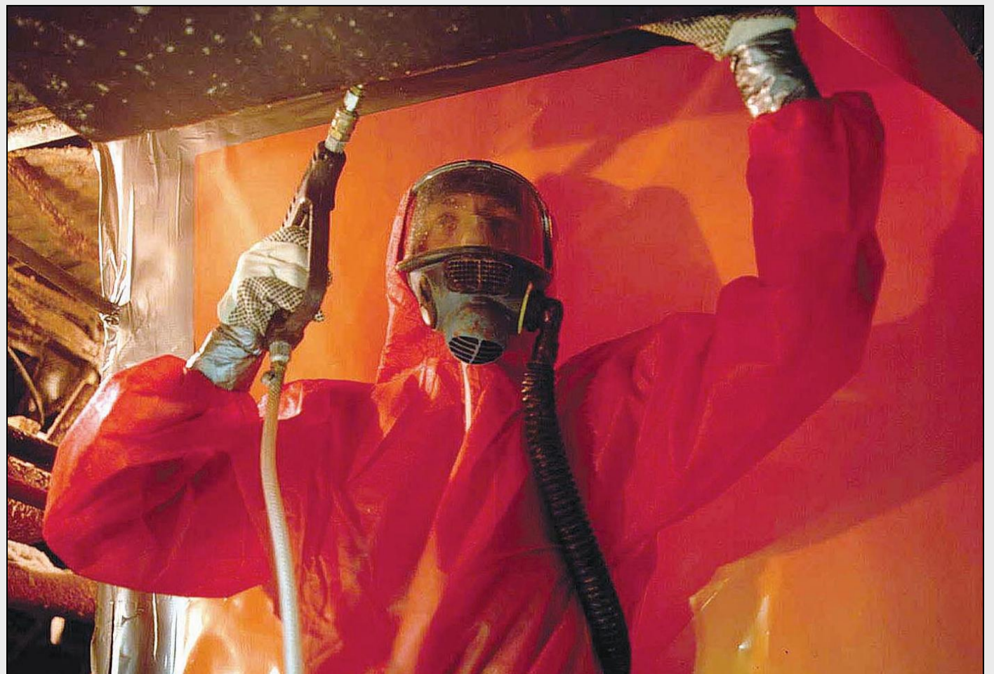
Asbestos removal: the commission is putting together a proposal that EU ships be sold to facilities with working practices on a par with the Hong Kong Convention.
